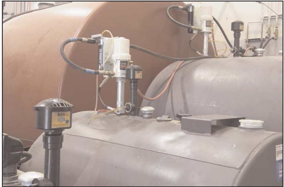
Tank leveling monitors, CleanLine™ filters and Fireball™ pumps transfer oil from tanks to nine banks of Graco hose reels and dispense meters serving 19 bays.
